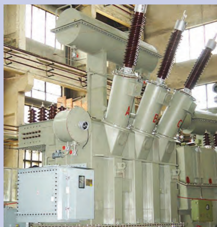
Transformer For Submerged Arc Furnace
