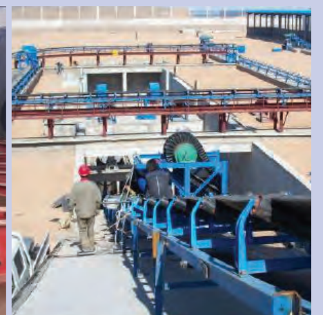
The Charging System
