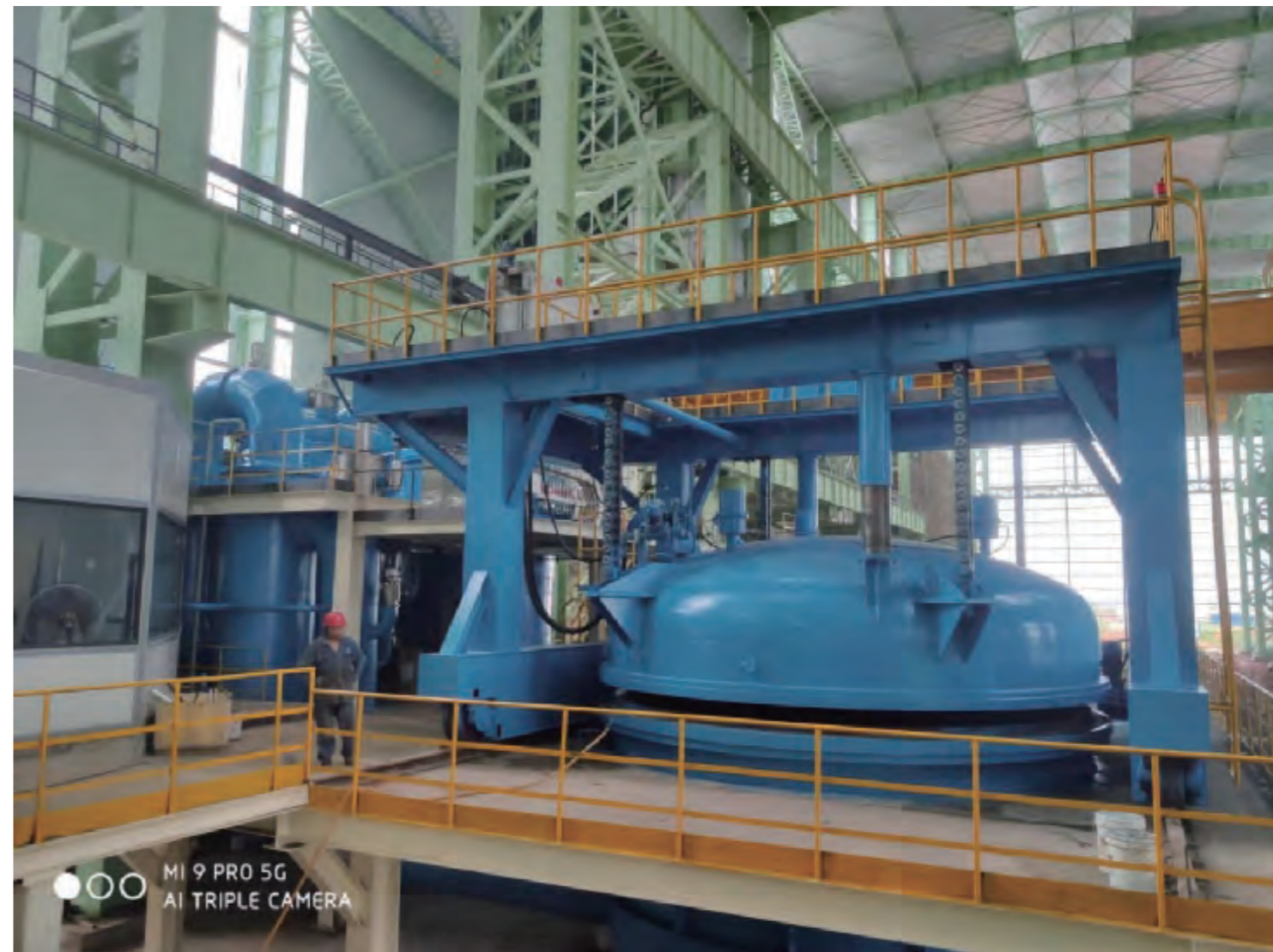
120t VD Vacuum Refining Furnace
