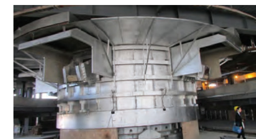
33000kVA Silicon Furnace
