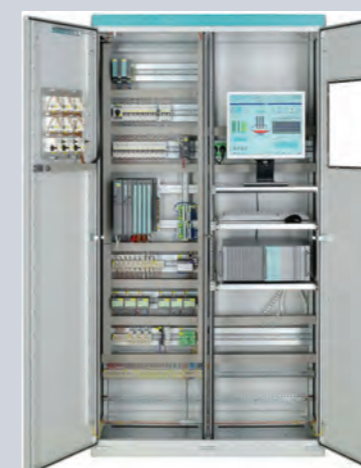
Electrode Control Cabinet
