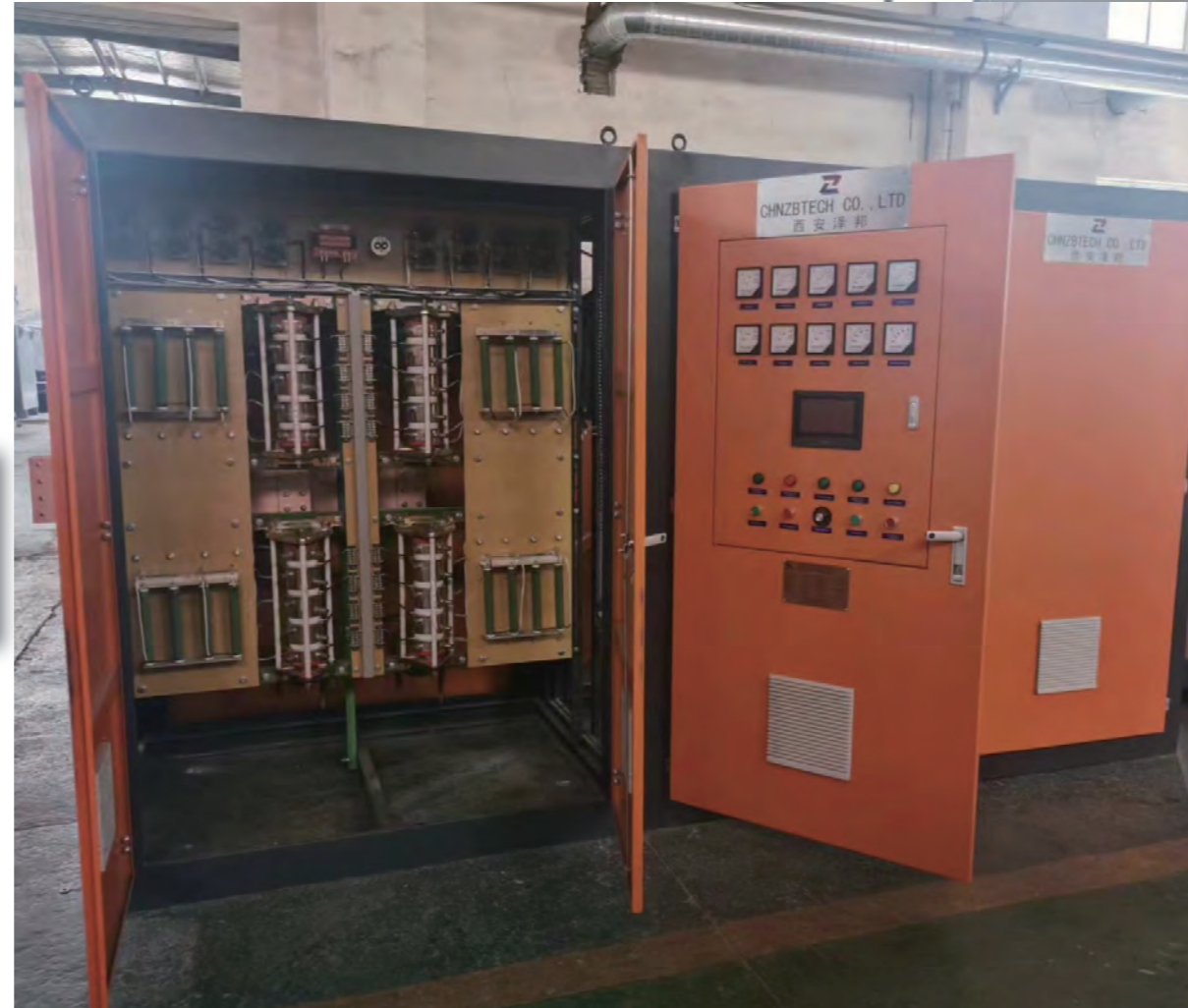
Electrical control cabinet of 20t IF induction furnace
