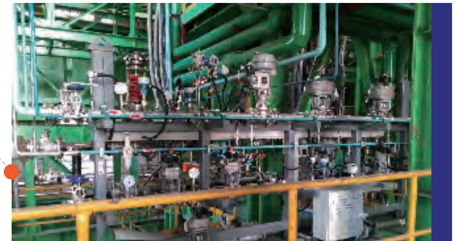
Oxygen Valve Station For EAF
