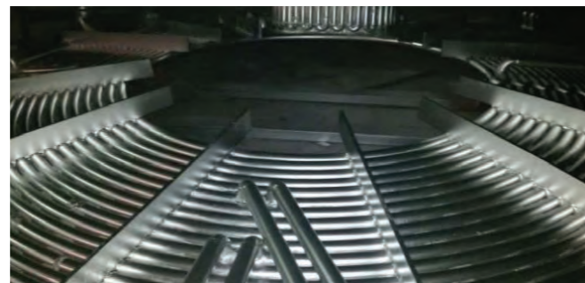
Cooling Pipe Furnace Roof
