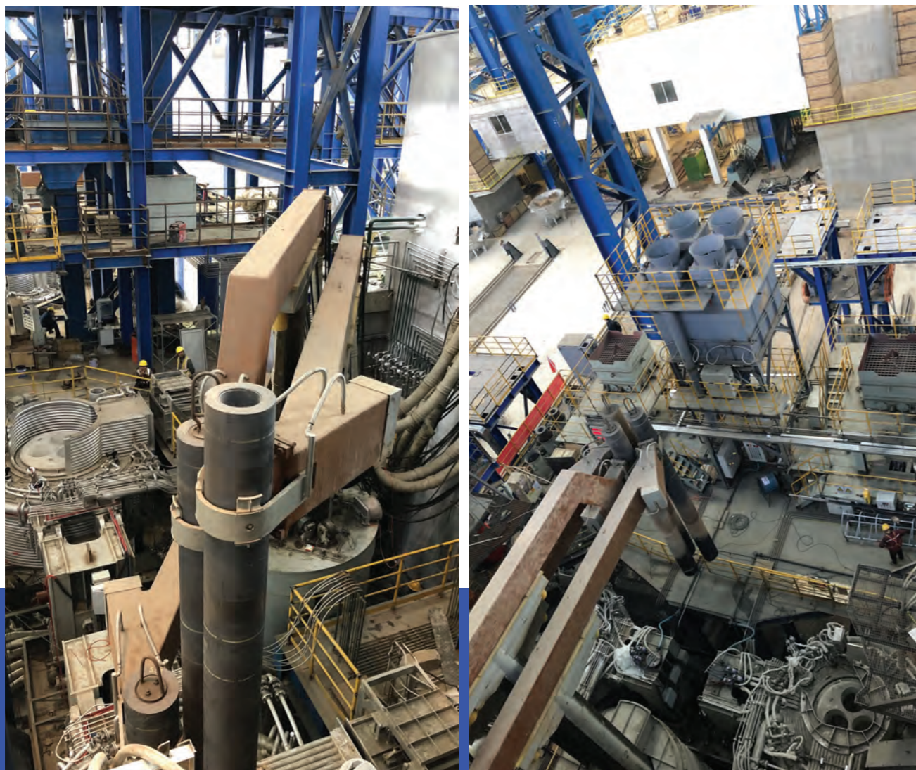
130t Ladle Furnace
