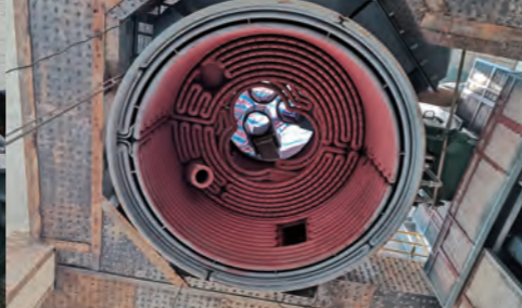
Water-cooled roof of LF
