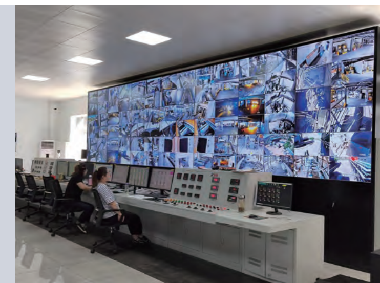
Monitored control system
